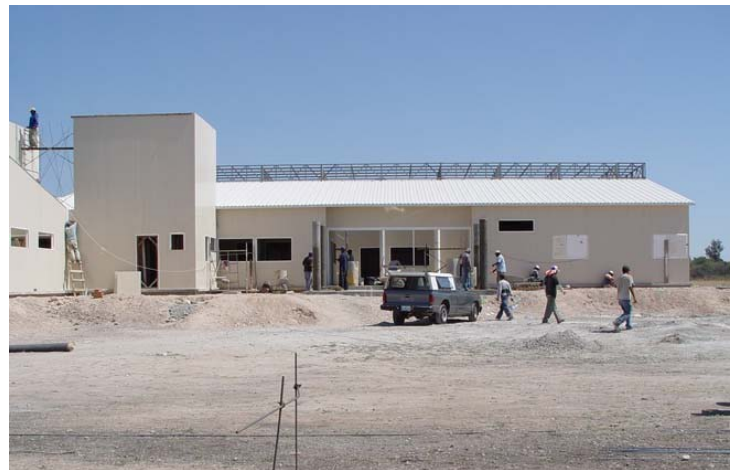
Construction of the new clinic is on track for a fall 2006 dedication
